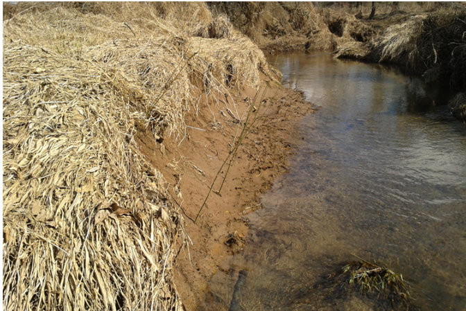
Exposed and eroding stream banks can be restored and stabilized through the practice of live staking.
